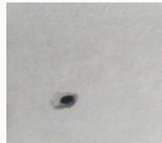
Figure 3: Hole on the ceiling made by the bullet.
