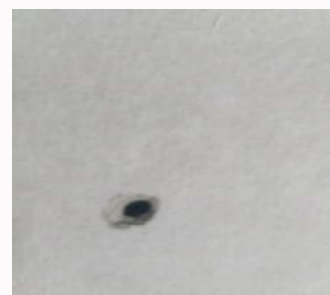
Figure 3: Hole on the ceiling made by the bullet.
